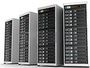
Primary Network Servers
